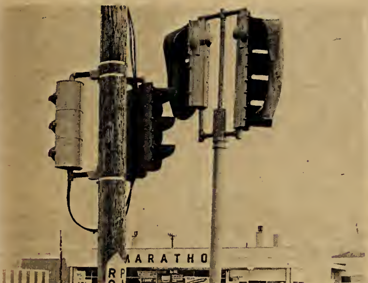
Meanwhile, a double set of traffic lights is located at Park and Roosevelt rd. Only one set is being used. -- Photos by Charles Andelbradt.
