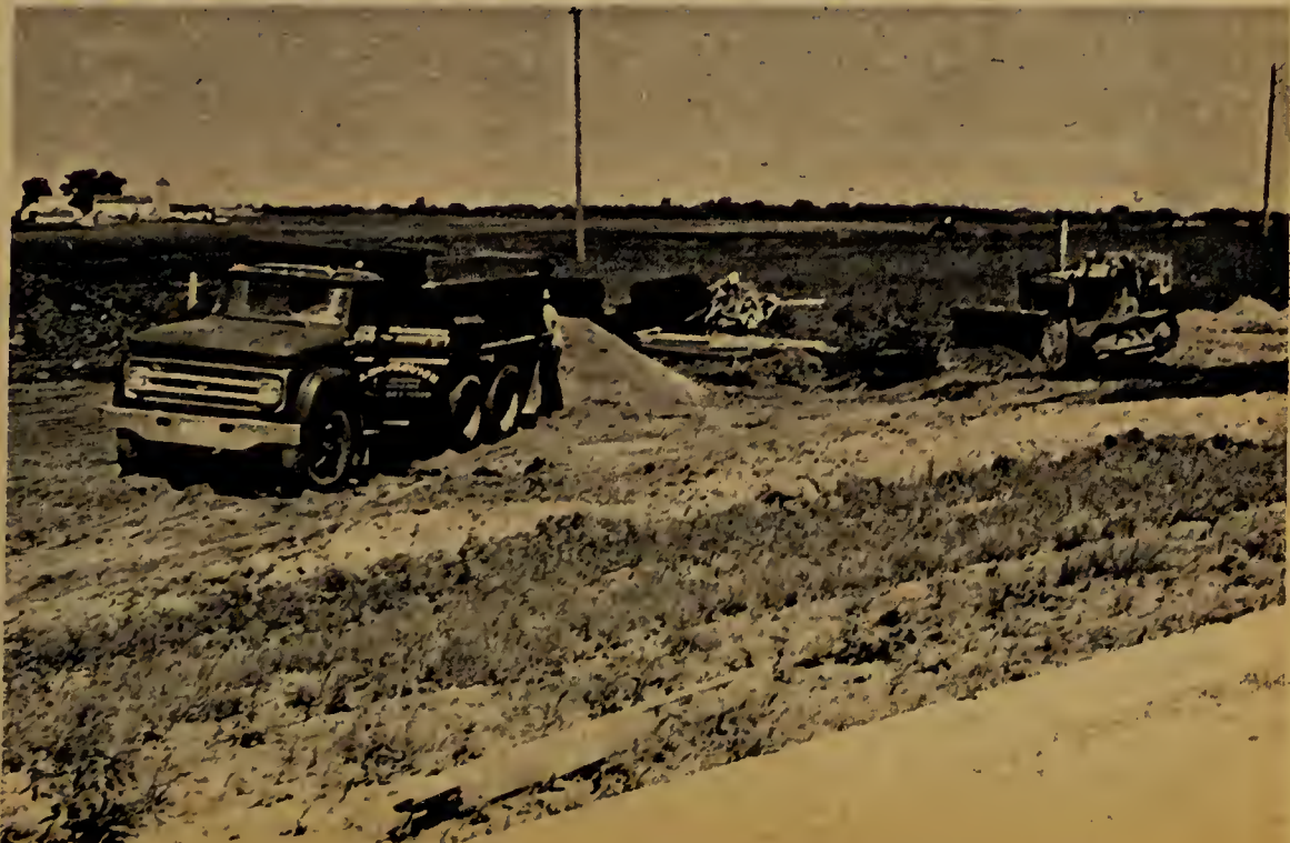
Bulldozer readies site for two new buildings at northwest corner of campus.
