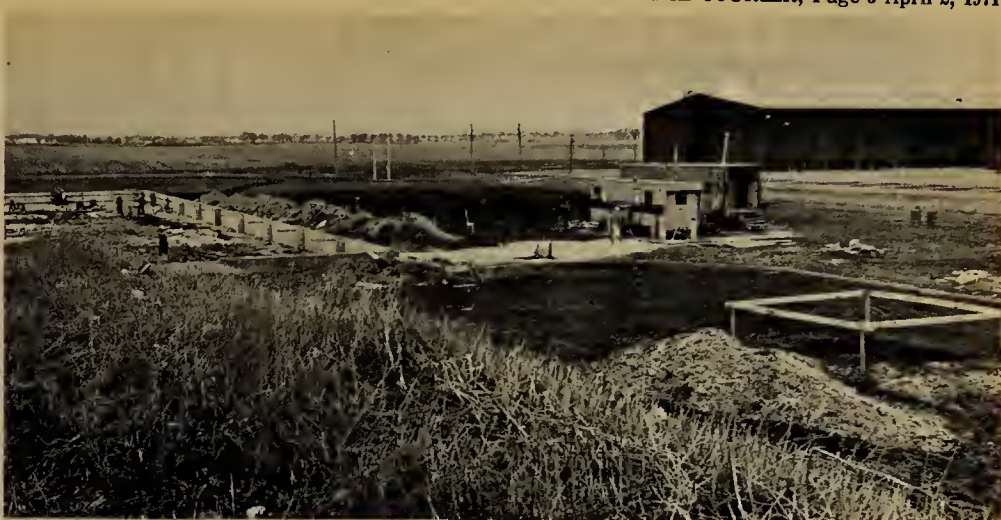
Construction progress is steadily moving along on 'M' Building, south of the main campus, a third large classroom structure scheduled for completion by September, 1971. Miller Davis Co. is handling construction of the building which is being built to alleviate increased enrollment next fall.
