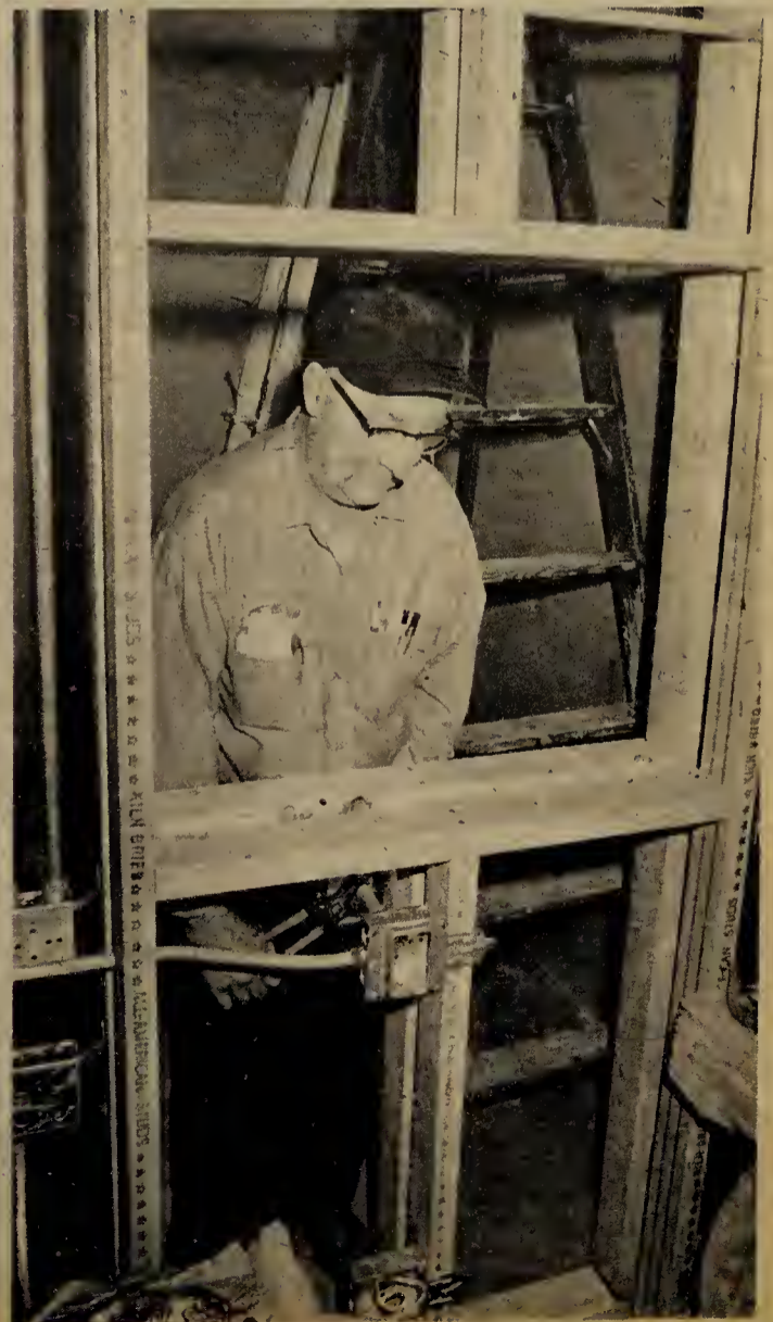
Quarters for the new radio station in J133, below, are beginning to take shape. Electrician Paul Vanderkoy, standing in the control room, looks into the small announcer's room.
