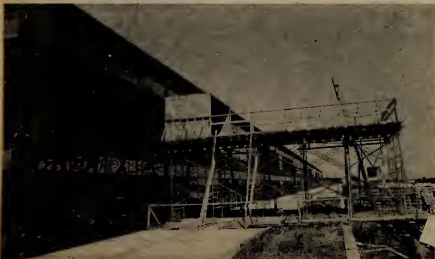
Persons new on campus usually ask: What are they building on the southwest corner of A Bldg.? The answer: that's a conveyor-hoist to get materials and equipment to the third floor, which is being outfitted for use in the winter.
