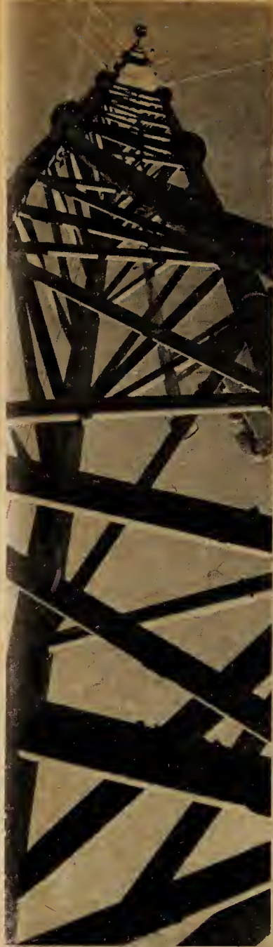
Up, up, UP! WDCB's 290-foot radio tower has finally arisen. The impressive structure towers over CD on the southwest corner of the campus near the tennis courts. WDCB hopes to go on the air sometime after the start of winter quarter. —Photo by Scott Salter.
