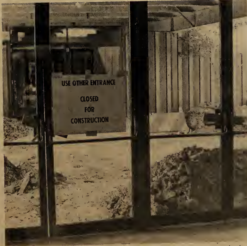
Construction between J and K buildings which is currently in progress, will eventually include new entrances, resurfaced walkways, and a permanent wall. The process should be completed by early October. Deliveries will have to be made with motorized carts, as no vehicles will be allowed on the walkways. — Photo by Maureen Murrin.
