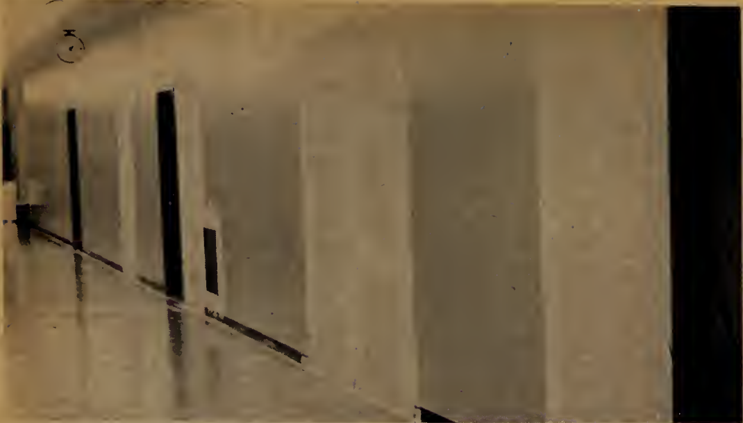
This may look like the work of some mad artist who likes to paint doors on walls — but actually it's the work of CD construction people who have been having a busy time sealing up some doors and putting in others in a hallway in J Bldg.
