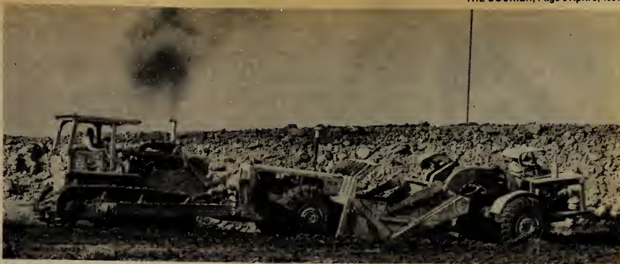
A giant earthmover gets a push in heavy going during SRC construction.
