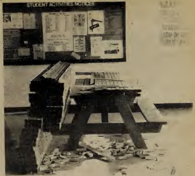
CLUTTER FROM INSULATION blocks second floor entranceway on northeast side of A Building. Insulation is expected to be completed by Oct. 15. COURIER photo by Roger Paulhus
