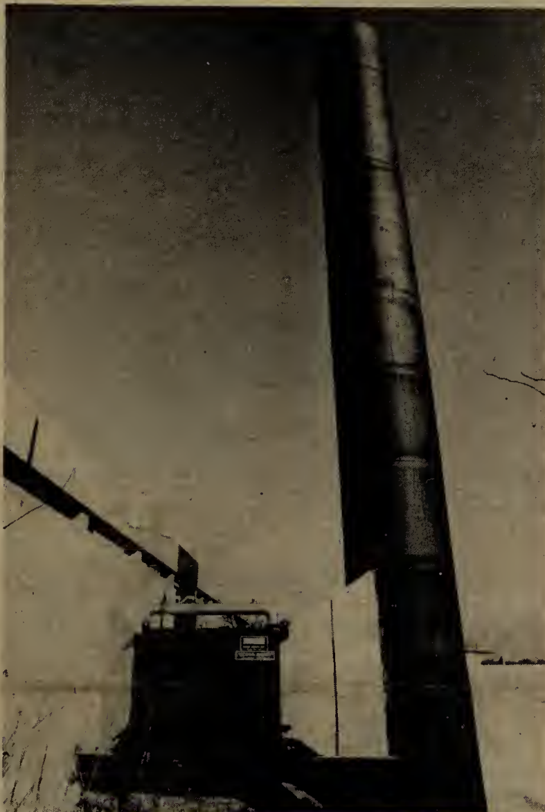
ECONOMIZER, LARGE BOX (left) was attached to chimney recently as part of energy-reduction program. Money-saving device makes use of otherwise wasted exhaust gases to preheat water condensing in system. COURIER photo by Ken Ford
