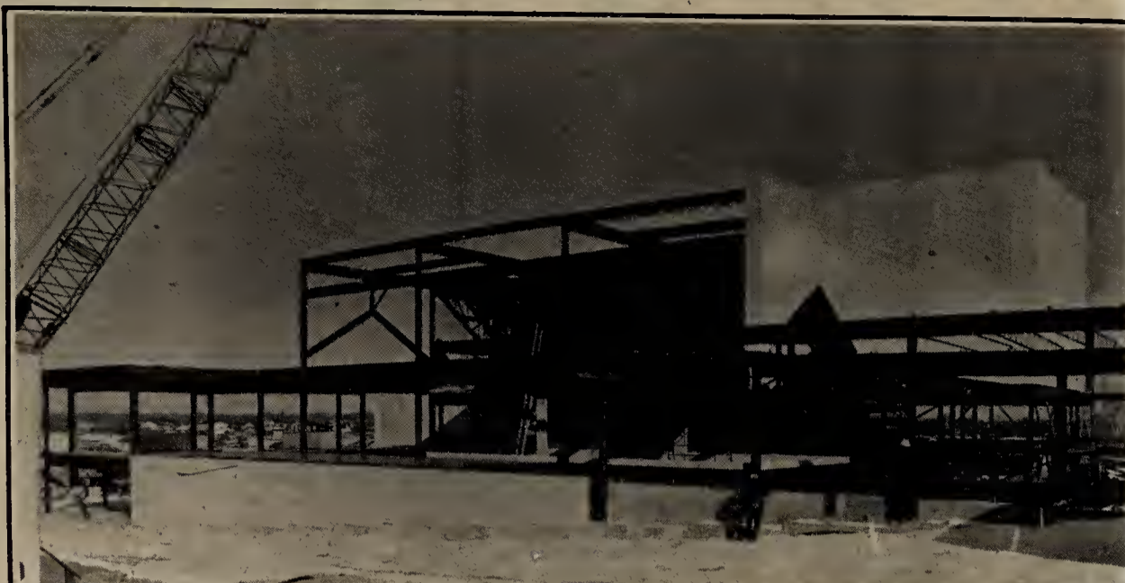
WORK CONTINUES ON Fine Arts Center, now estimated to be 35 percent complete. Delays incurred by bad weather have caused construction to fall 28 days behind schedule.
