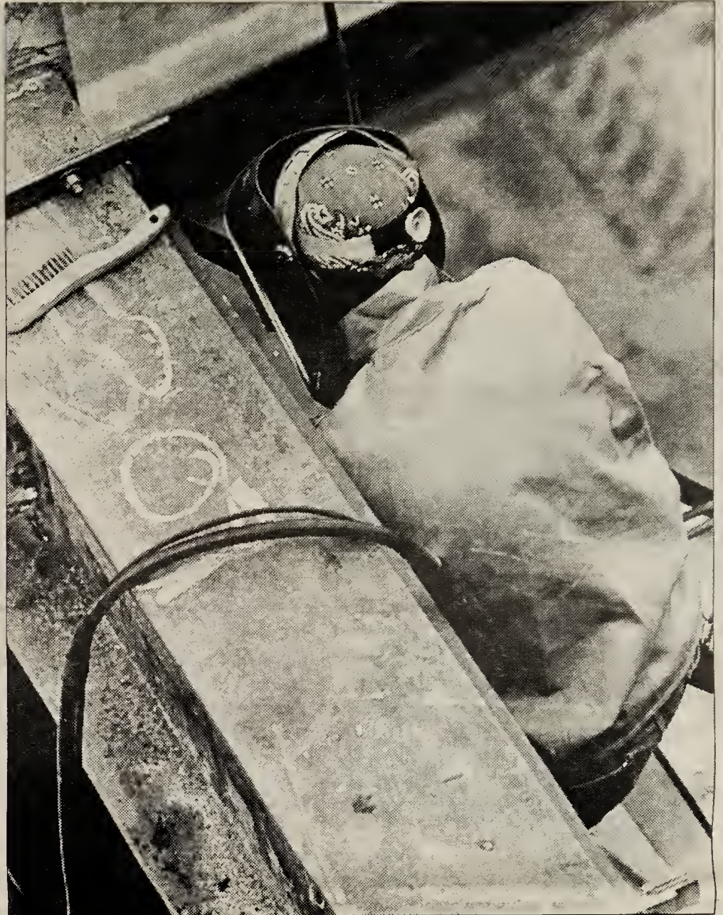
Wearing a welding mask, a construction worker prepares to weld a girder.
