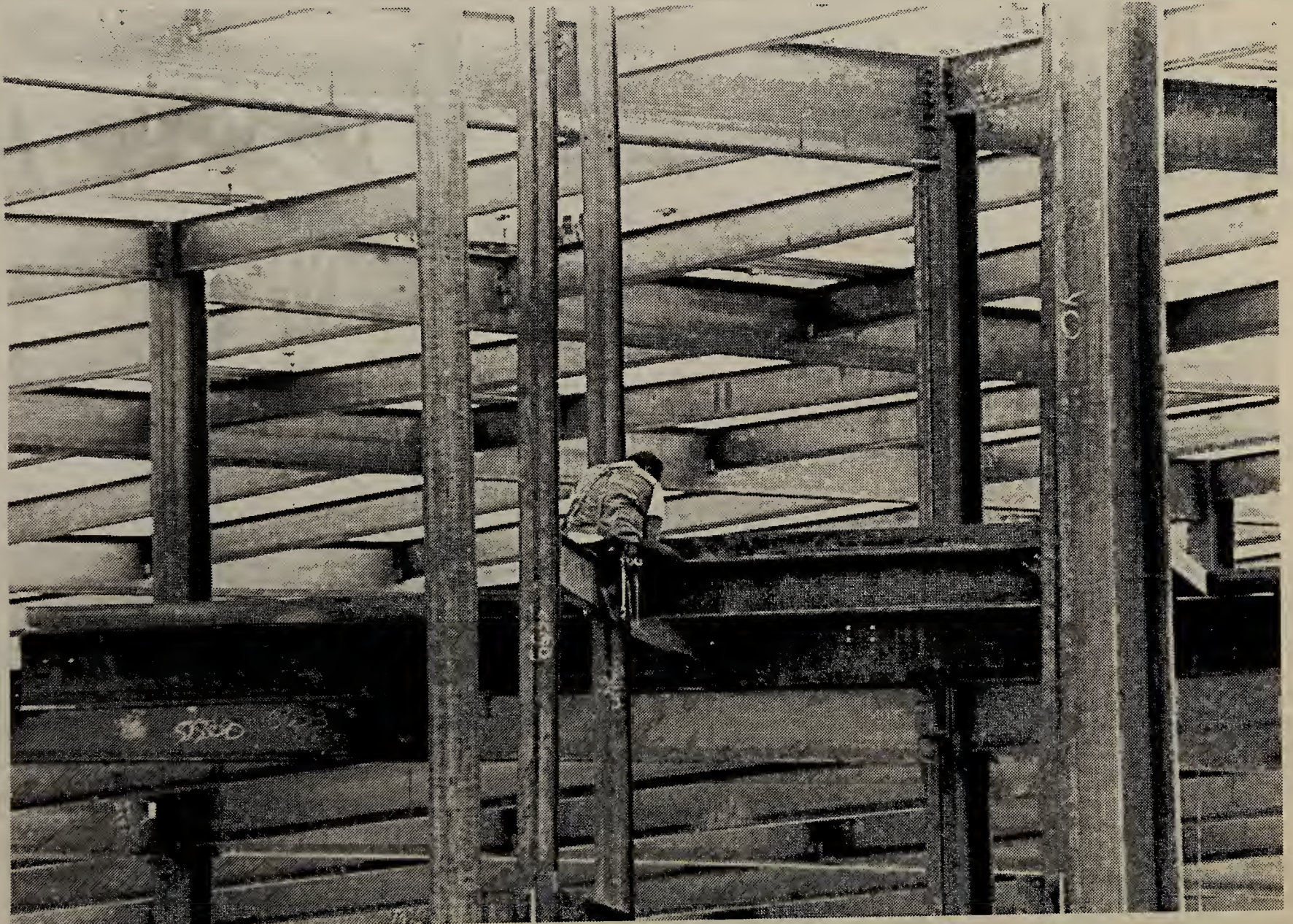
Perched like a bird, a construction worker prepares a girder for welding.
